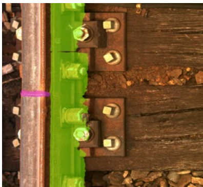
Rail insulated joint detected
